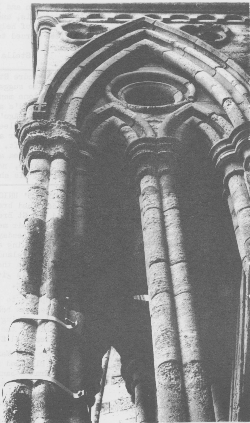
A fractured stone in a gablet of the Central Tower which has been temporarily restrained with metal straps and will have to be replaced completely. The deterioration of the stonework and an earlier repair with a cement mixture can be clearly seen.
